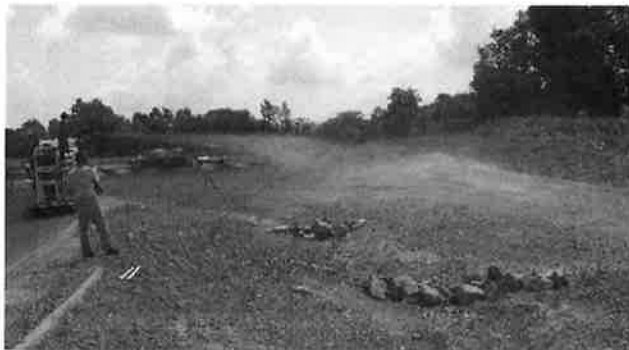
Hydraulically applied seed, mulch, tackifier, and soil amendments (e.g., lime, fertilizer) offer excellent results at a reasonable price on large sites, especially those with long, steep slopes. Follow manufacturer's recommendation regarding materials mixing and application rates.
