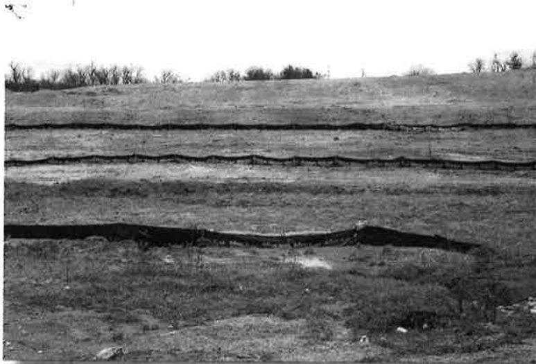
Use multiple silt fences at proper spacing (see table) to protect long, unvegetated slopes. Fences provide only temporary protection and can be removed when the area is seeded and mulched.
