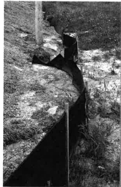
Silt fence is functioning well, but needs maintenance. Set fences back from the toe of the slope, to allow room for sediment to accumulate and maintenance.
