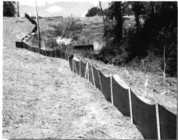
Silt fence installed backwards—note that stakes are on the uphill, rather than downhill, side of the fabric. Ponding flows against this fence will push the fabric away from the stakes, causing failure and releasing sediment to the small stream on the right.
